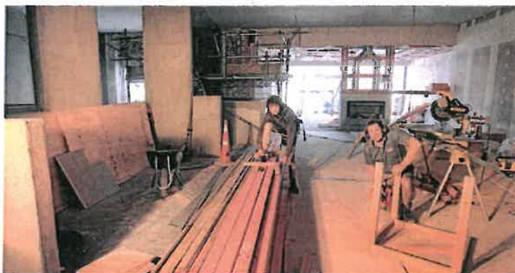
Substantial building work requires a good contract so both parties have a clear understanding of the terms and conditions.
